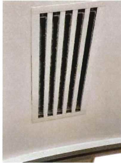
Figure 2: Clean return air vent in vending area
