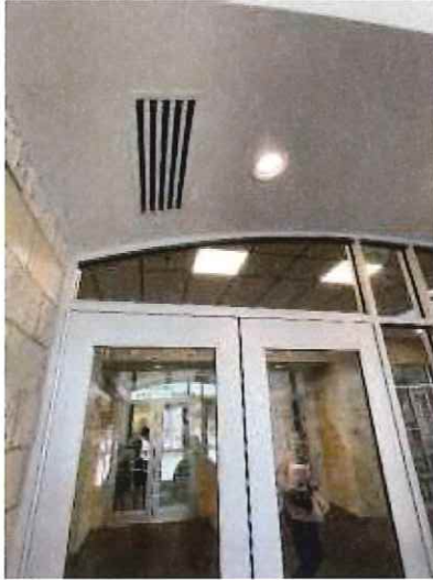
Figure 1: Install glass missing from storefront
